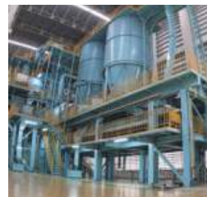
Sand conditioning system
